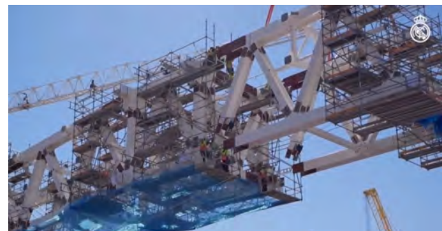
THIS IS HOW THE TRANSFORMATION OF THE SANTIAGO BERNABÉU STADIUM IS PROGRESSING
