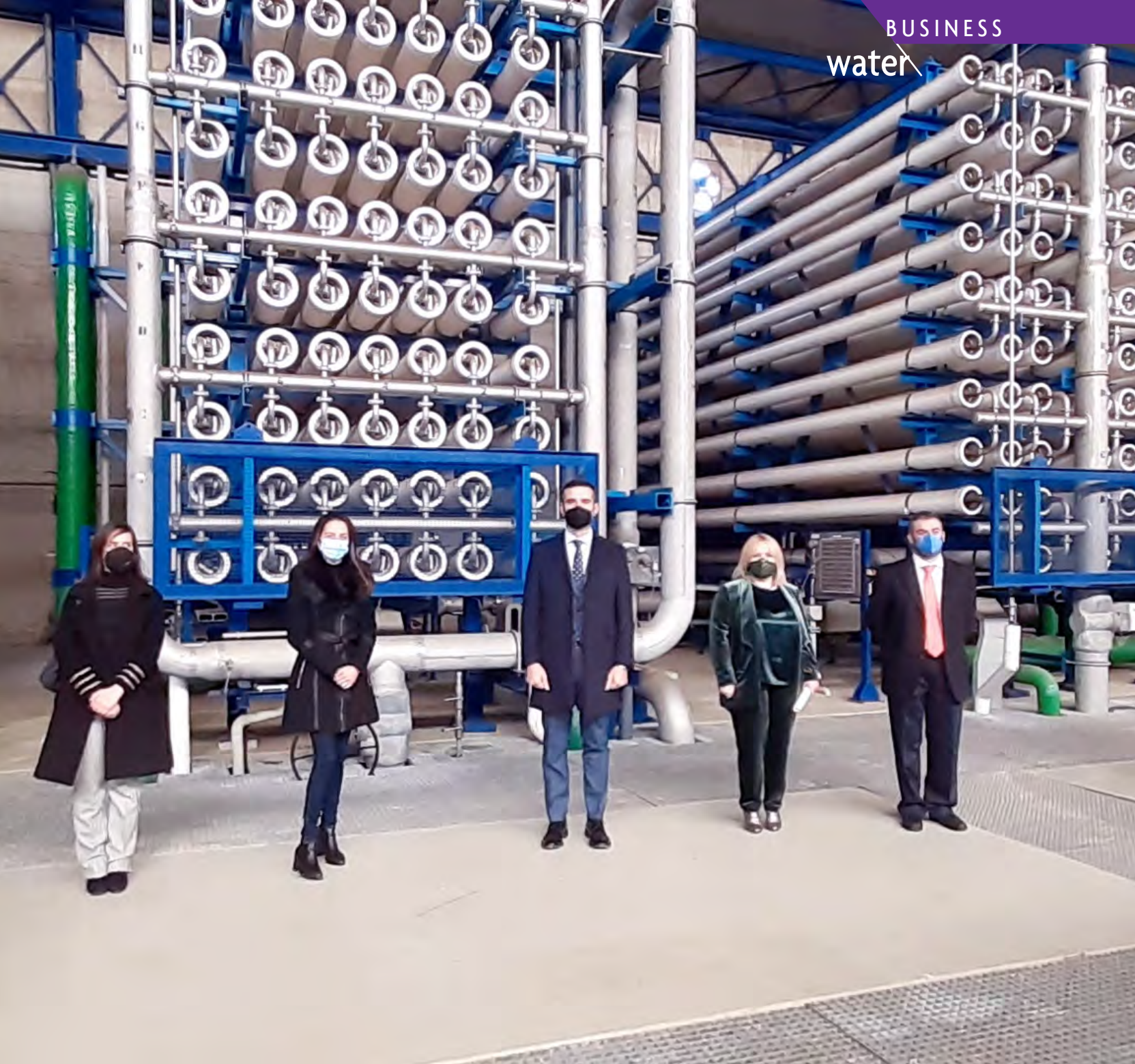
Government of Andalusia visited the former Rambla Morales desalination plant, now Mar de Alborán, in Almería.
